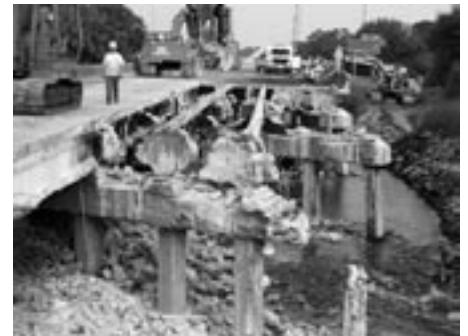
When the Big Slough crash happened, construction teams immediately went to work.
