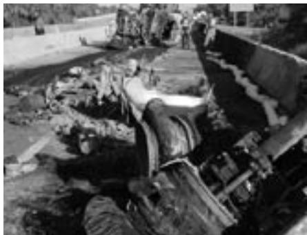
The gasoline spill and cleanup kept crews from getting a close look underneath. But what they could see was devastating.
